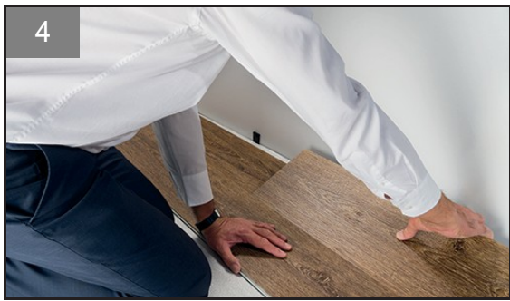
Figure 4: Working from the wall, insert plank 3 into the long side of plank 2.
